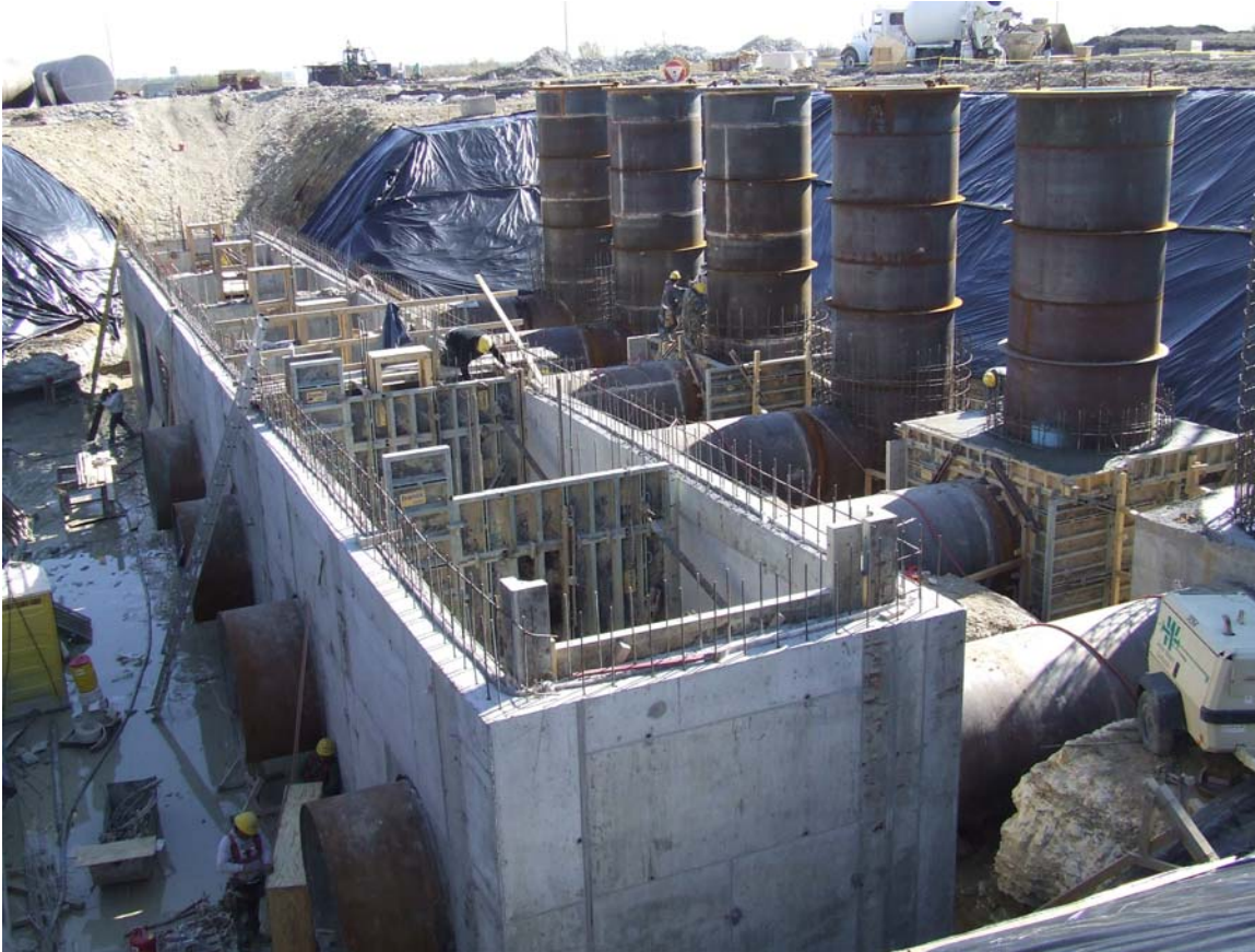
Figure 2. Rolling Hills BPS Suction Valve Isolation Vault and Pump Barrels
