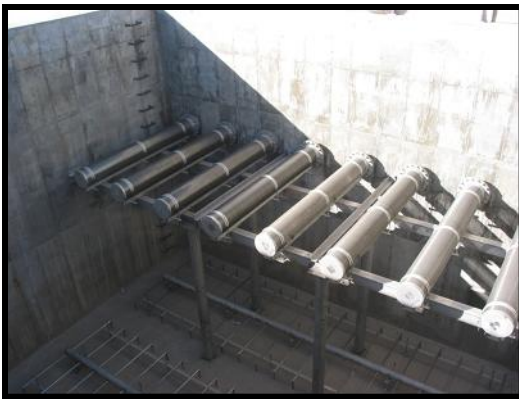
Figure 8 Circular Wedge Wire Sieve Installation
