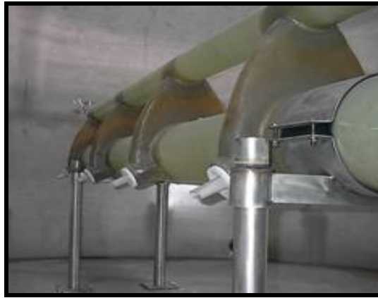
Figure 7 Slot Injector Aeration System
