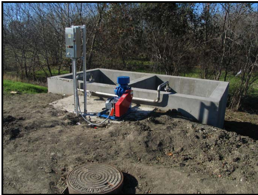
Figure 10 MBBR Reactors with Positive Displacement Type Aeration Blower
