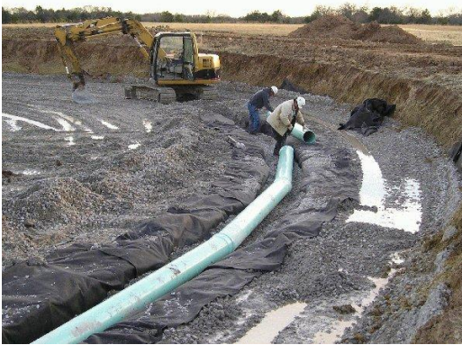
Photo 1. 6 MG tank perimeter drain piping
