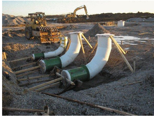
Photo 2. 6 MG tank overflow piping
