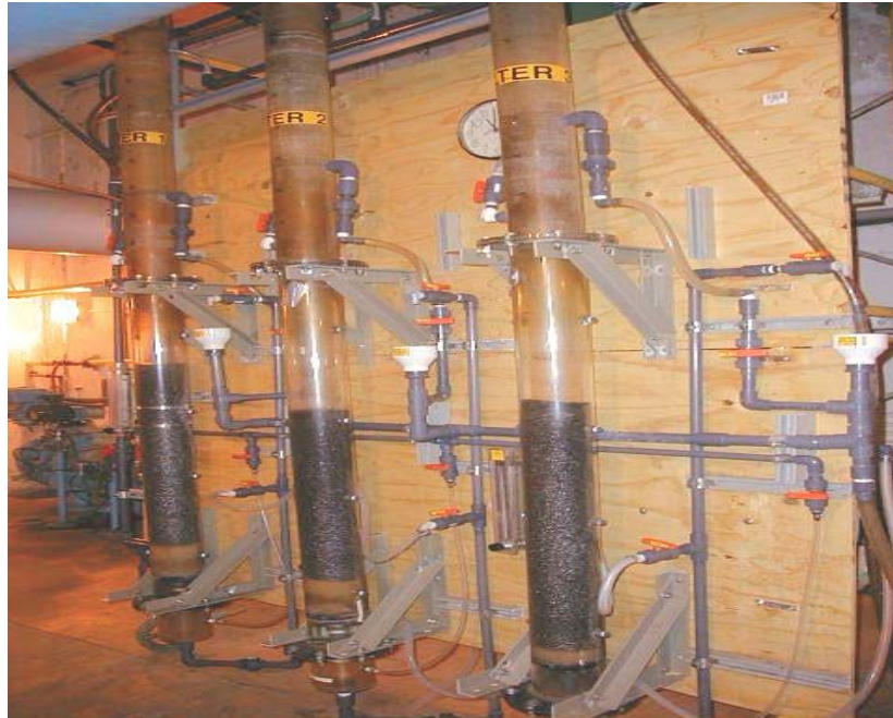
Figure 2. PBS Pilot Plant Photo
