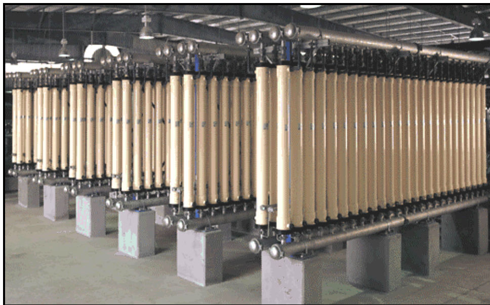
Figure 2: Pall Pressurized Membrane Installation
