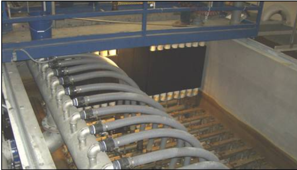
Figure 3: Siemens Vacuum Membrane Installation
